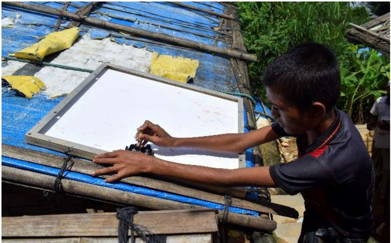
A newly trained young boys is repairing solar panel in the Rohungya house as a daily wage basis.
